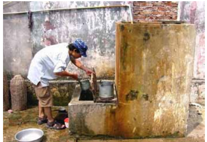
Above: Sand filter for iron and arsenic removal, used by rural households in the Red River delta (Vietnam). Photo: copyright Eawag
